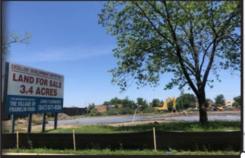
Engineering was completed to prepare new shovel-ready sites at Grand and Mannheim for retail and commercial redevelopment.
