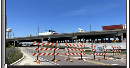
Phase 2 of the Franklin Avenue Reconstruction Project has begun with work to allow for additional lanes at the I-294 underpass.
