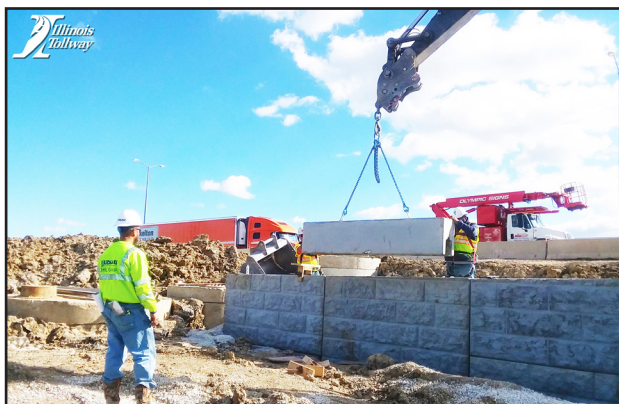
Tollway improvements occurred in Franklin Park in advance of the I-490/I-294 Tollway Interchange construction (Image courtesy of the Illinois Tollway, 10/2018).
